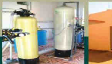
RO Plant Batch 1982-89 (2007)
